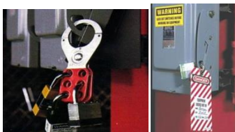
Locks and tags for electrical panels
