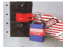
Breaker switch lock and tag
